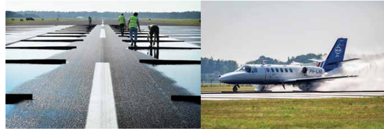
On the left: waterpond construction at Twente Airport On the right: aircraft in flight testing
